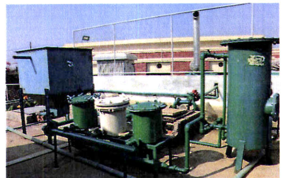
Sewage Treatment Plants (STP) at the campus
